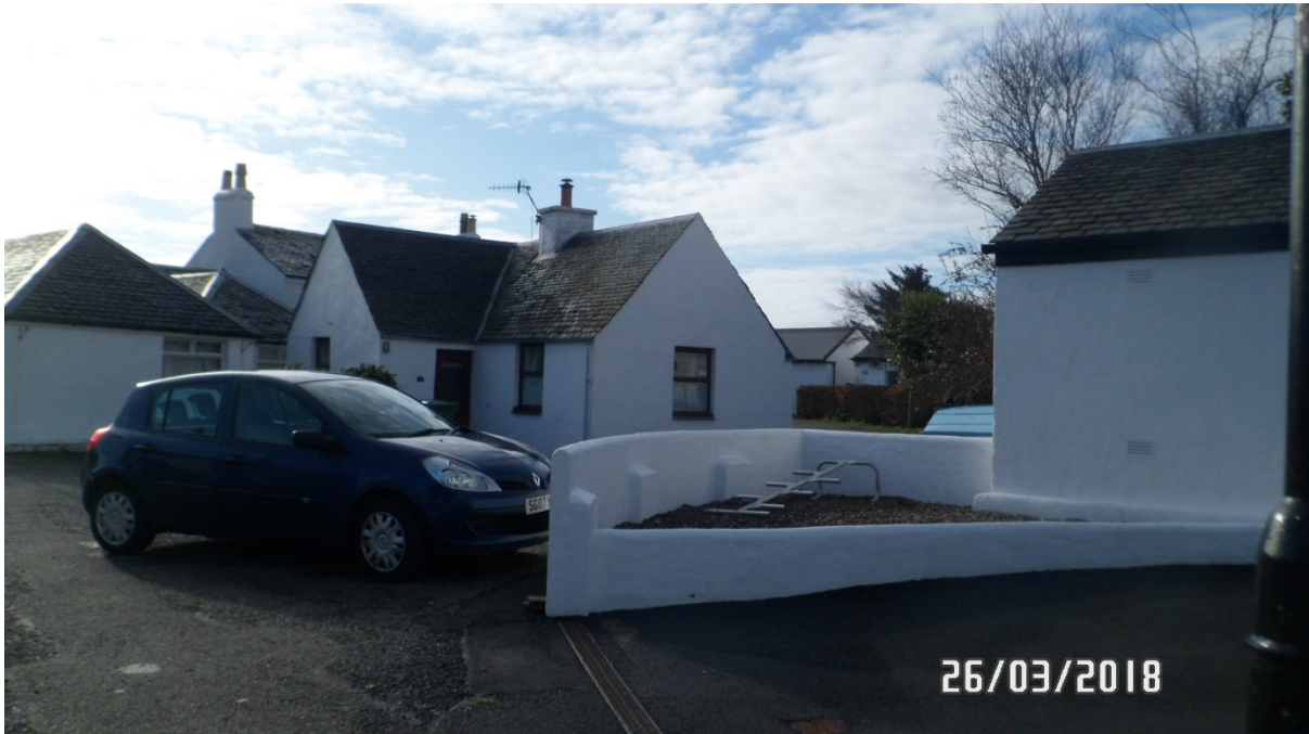
Front elevation showing 3 no. brown painted timber top hung windows and brown painted timber half glazed entrance door
