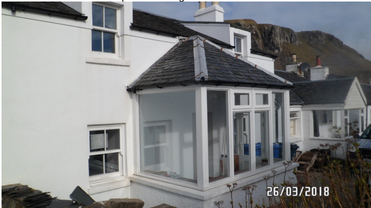
Front elevation showing white timber sliding sash and case windows to ground and first floors and entrance porch with timber windows and timber entrance porch
