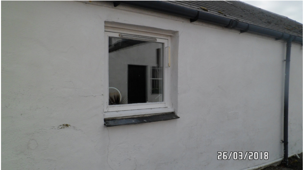
Close up showing white painted timber side opening unit to rear elevation
