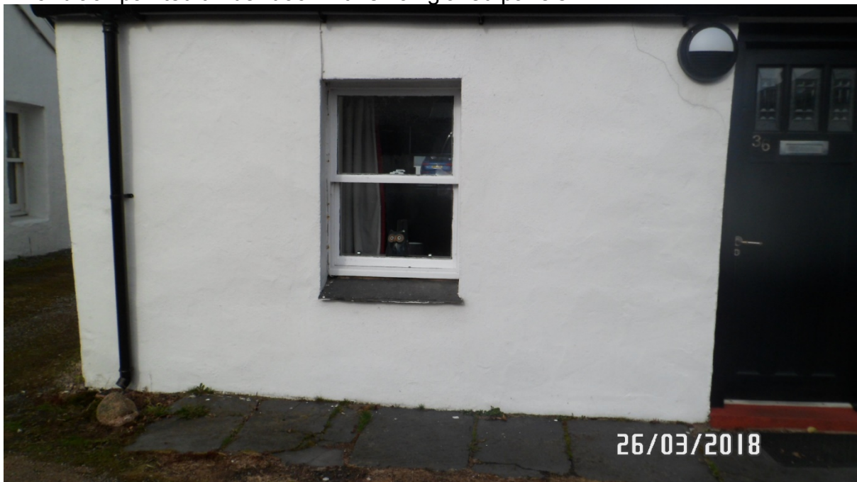
Close up of white painted timber sliding sash and case window to front elevation
