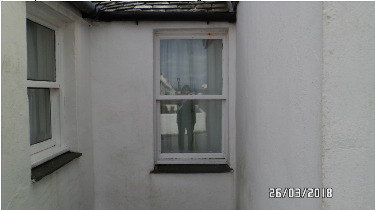
Close up of single white painted timber sliding sash and case window to rear elevation
