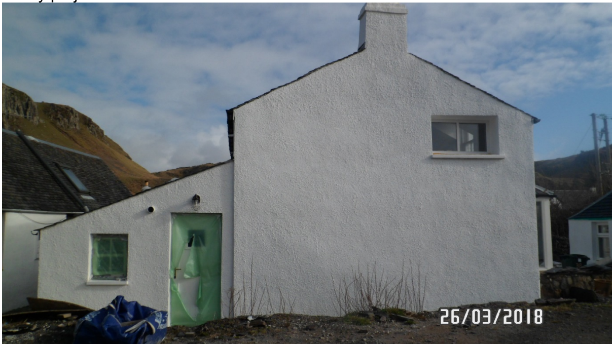
Side elevation showing 1 no. white painted timber unit at first floor the method of opening of which is not clear with 1 no. white painted timber door with glazing panel and 1 no. four pane white timber window to the side elevation of the single storey rear projection the method of opening of which is not clear.
