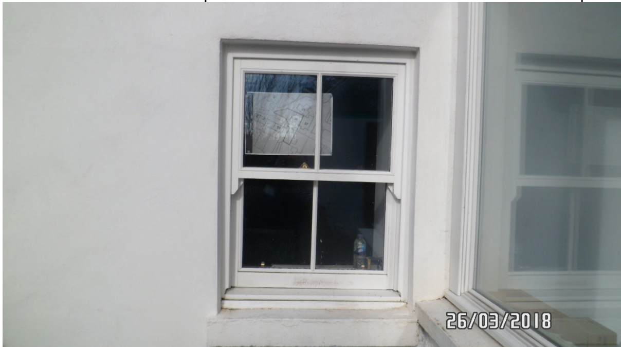
Close up of ground floor white timber sliding sash and case window to left of entrance porch
