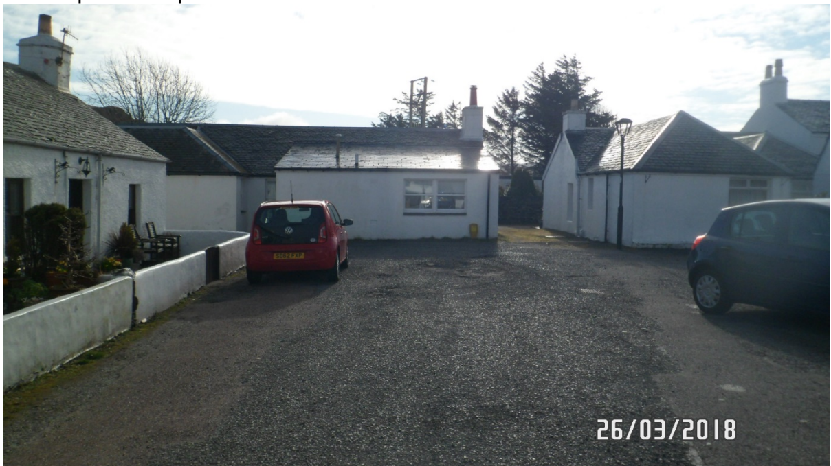
Rear elevation showing 2 no. white painted timber sliding sash and case windows, one double unit and one single unit
